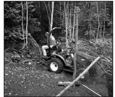
Jerry Fehrmann fires up his tractor at the clubhouse and digs improved drainage for the shooting and archery ranges.
