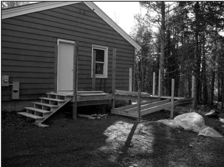
New clubhouse deck and entry ramp shown under construction has been completed thanks to the carpentry of Johnny Johnson and Tom Kehoe.
