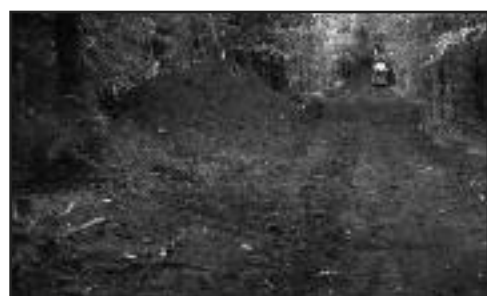
Shooting sports facilities make progress as multi-purpose shooting lanes for archery and guns are bulldozed through the woods.
